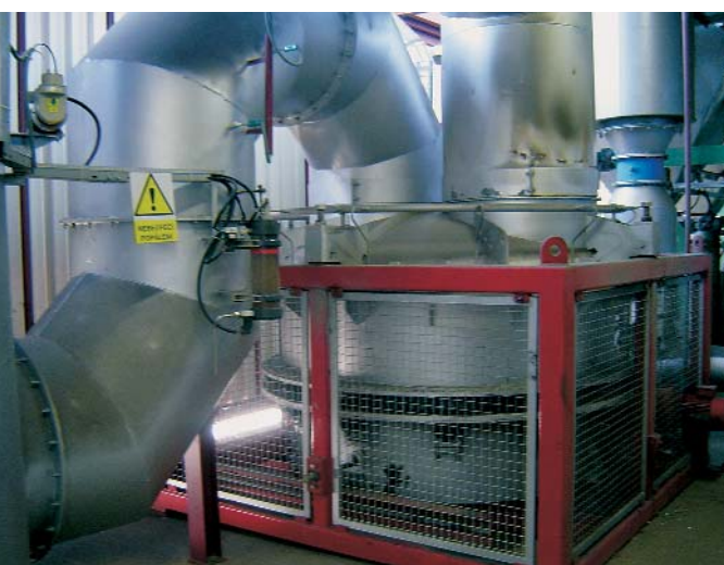
Fig. 3: Heat recovery behind the thermal post combustion by an EcoReg®
